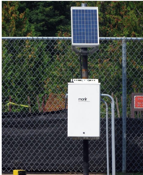
Datalogger powered by the solar panel installed at Bolsover Dam
