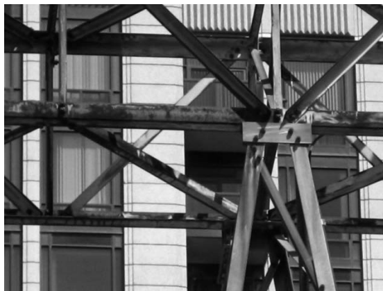
Figure 4 Some typical bolts used as monitoring points (Monir Precision Monitoring, 2008)
