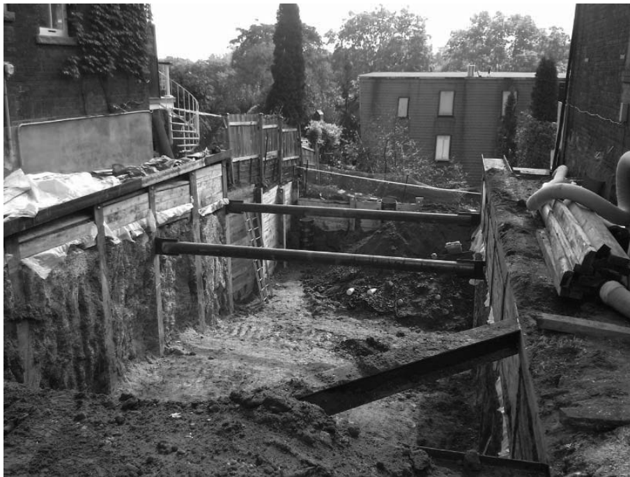
Figure 11 The excavation and the two buildings being monitored (Monir Precision Monitoring, August 2014)
