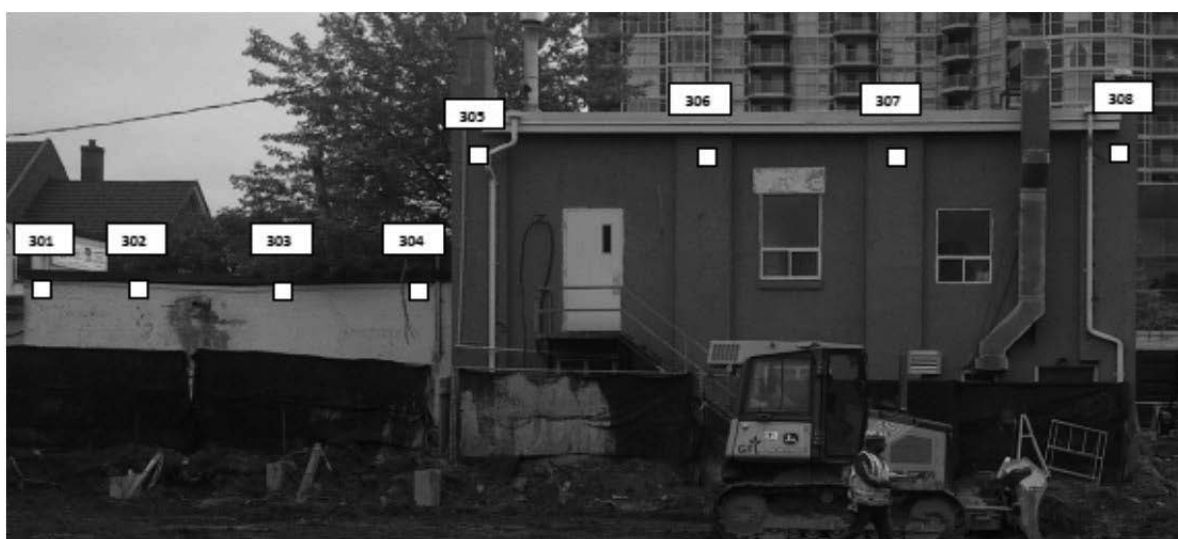
Figure 8 Monitoring locations on some of the unreceptive buildings (Monir Precision Monitoring, February 2012)
